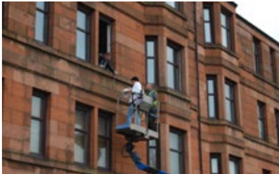
The Italian partner RED installing equipment for heat-flow measurements of the aerogel retro-fitted wall in the Glasgow tenement case study (Photo: Historic Environment Scotland)
