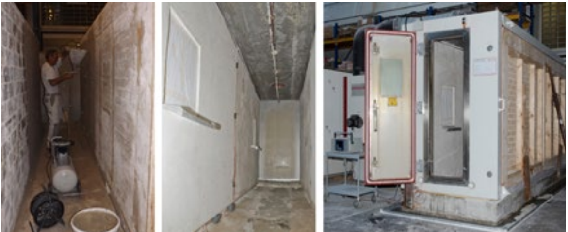
Spray application of insulating lime render on a wall forming the enclosure of a climate chamber (Photo: MPA Stuttgart)
